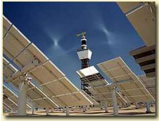
Power tower system
