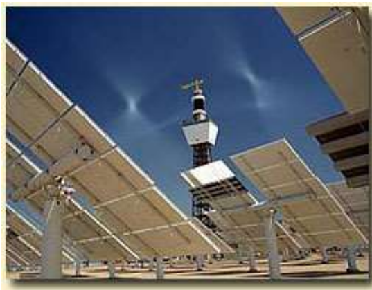
Power tower system
